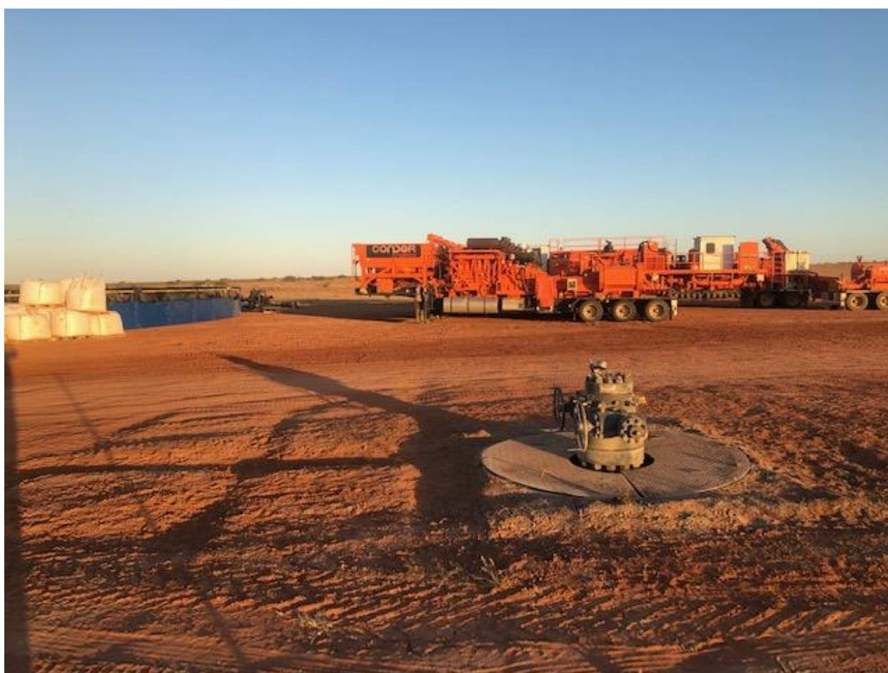
Figure 2: Vali-1 ST1 well head and Condor Energy Services equipment
